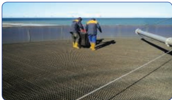
Tough stuff: Trickling filter media made from polypropylene need no protective grating to prevent damage during inspection
